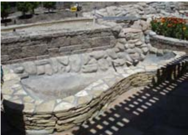
The pond is complete and ready for water. He can't fill it until he has gates installed for compliance to building codes. The pond has cement lining and stone walls. Dry laid concrete masonry units across the back are part of the retaining wall.
