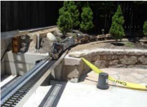
Using two aluminum angles to form a temporary crossing makes it possible to get track laid before completing the bridges.
