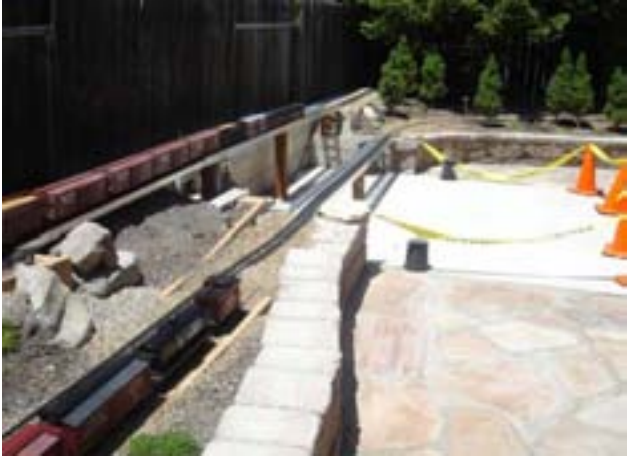
Work is still going on here. The tape outlines where a storage shed will be built to house the trains. This is the side yard looking toward the corner of the backyard.
