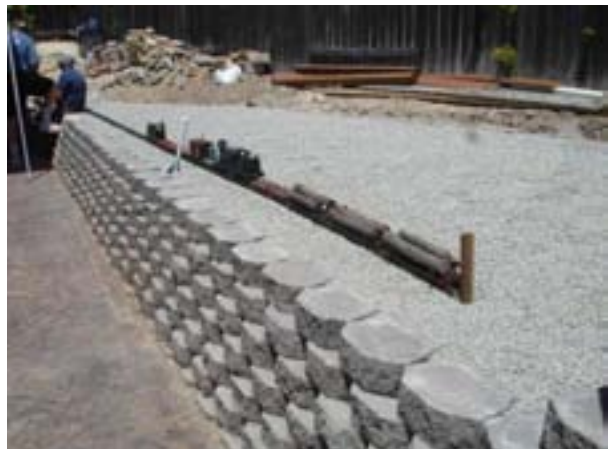
This is the newest part of the railroad along the other side yard. This area will be developed as a rail yard. A good example of dry-laid, interlocking concrete blocks. This track, put down two days before the open house, still has to have a roadbed with ballast.
